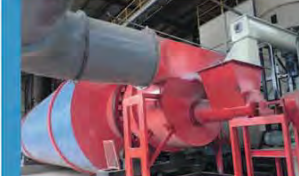
Rotary Drum Dryer 09
